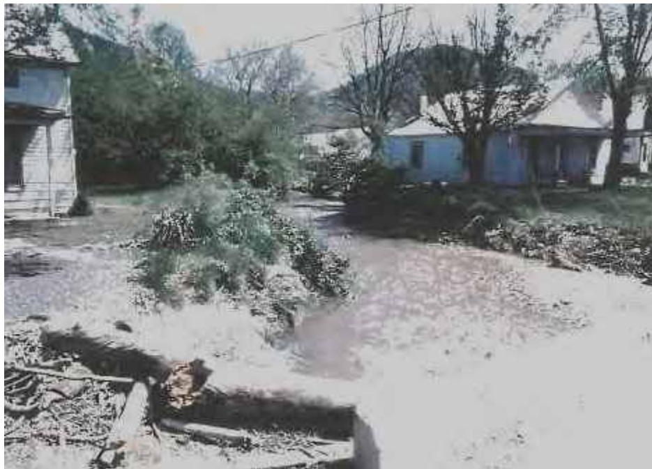
Debris and Sediment Blocking Street Culvert Opening (bottom left) Near Confluence of Noel's and Indian Gap Runs after April 1992 Flood
