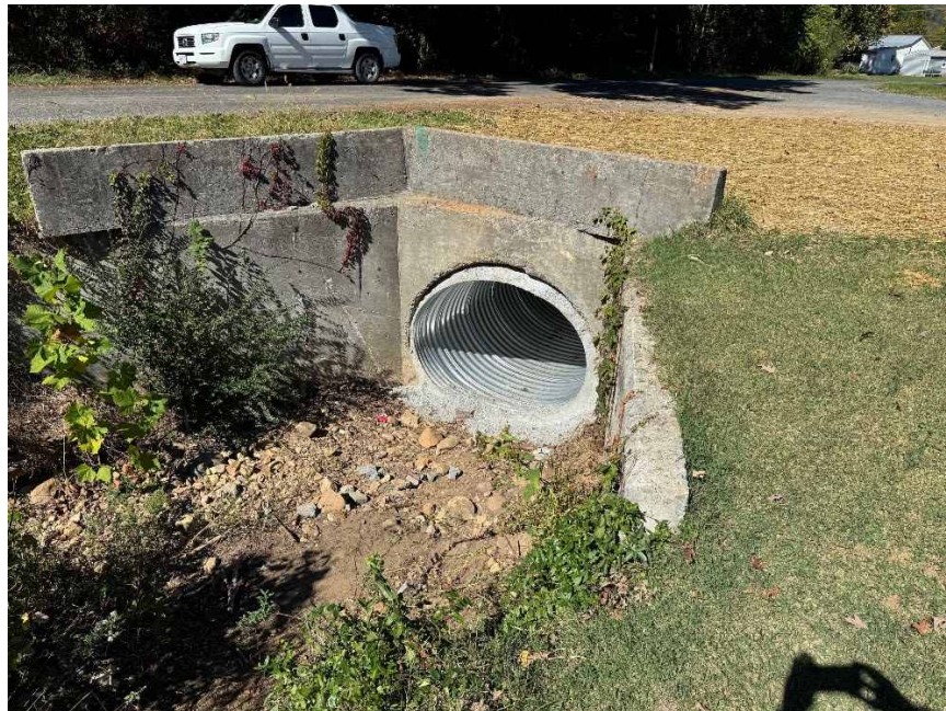
Top: Failed Entrance Prior to Temporary Repair Bottom: Temporary Repair (10' of replacement pipe at entrance)
