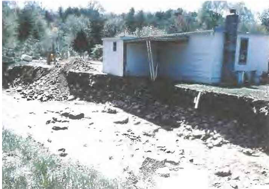
Scouring of Stream Channel on Pedlar Gap Run after April 1992 flooding
