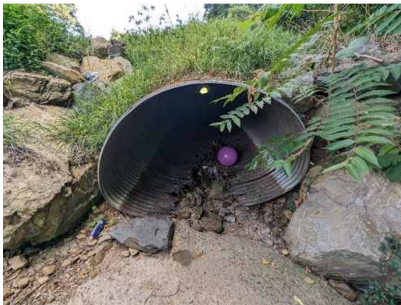
Outlet Showing Complete Absence of Pipe Bottom for Entire Length
