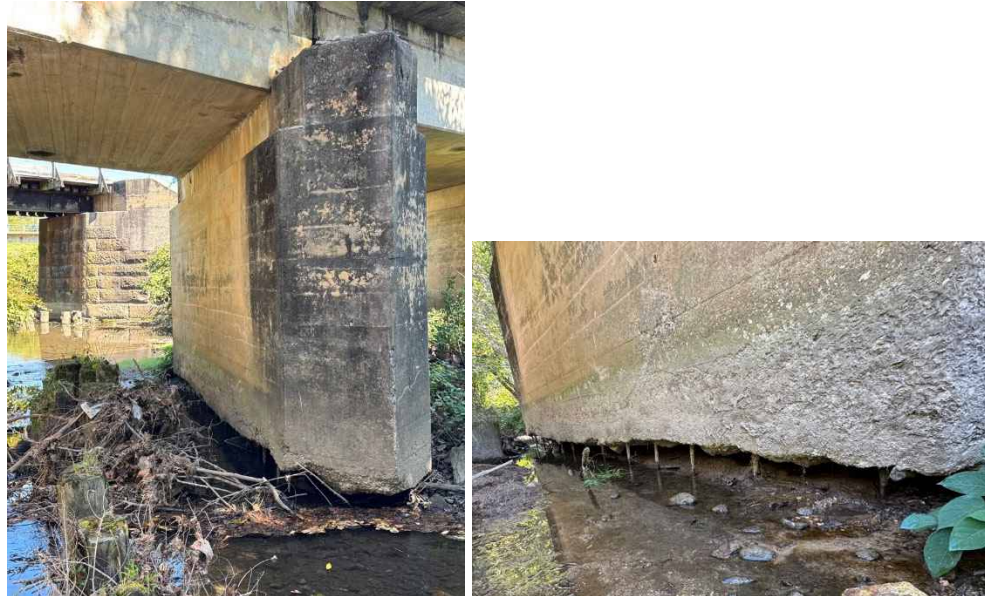
Scour Under Pier of Upstream Railroad Bridge (set for repair)
