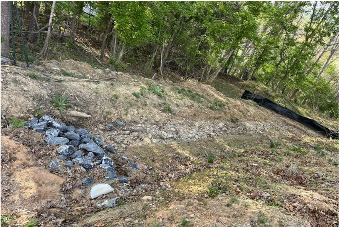
Storm drain ditch on south side of 32nd St; 32nd St at left outside image, termination at silt fence at right
