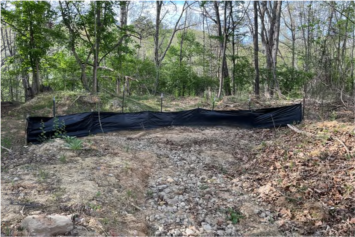
Silt fence where drainage ditch currently terminates; Chalk Mine Run just past trees
