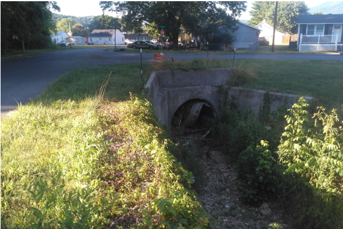
EAST SIDE OF WOODLAND AVE CULVERT INLET SHOWING COLLAPSE
