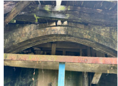
Section M: Failed brick masonry arch.
