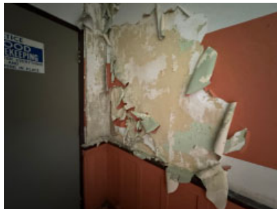
Section D: Office wall finish deterioration.
