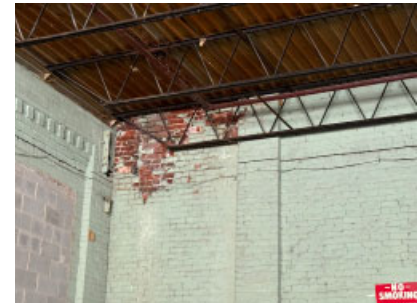
Section C: Southwest corner masonry condition.
