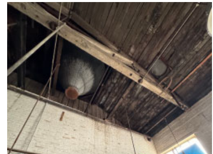
Section B: Room 4 through-roof tank.
