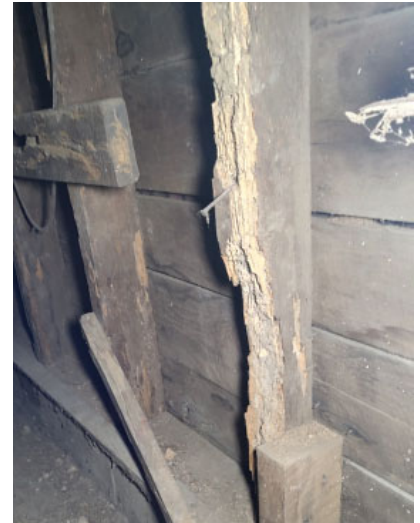
Building X: Termite damage at wood studs.
