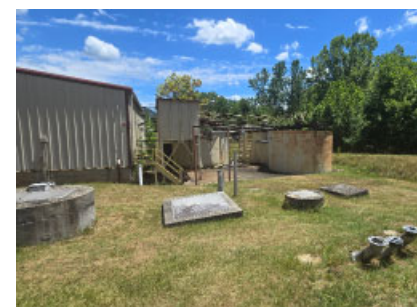
On-site water treatment plant.
