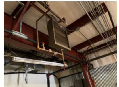
Section A: Gas heater.
