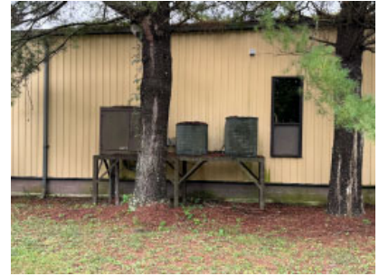
Section A: Air conditioning units, north side of structure.
