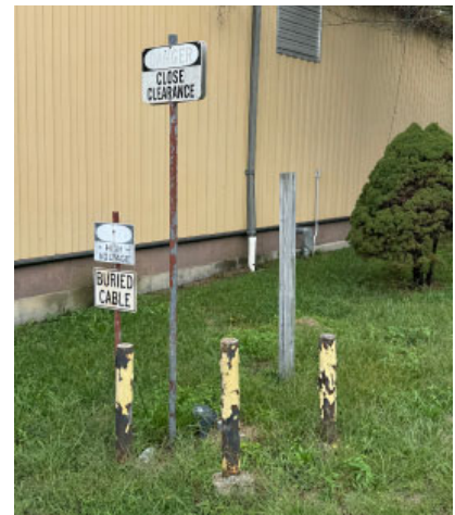
Section A, north side: Buried cable signs opposite the former transformer yard.
