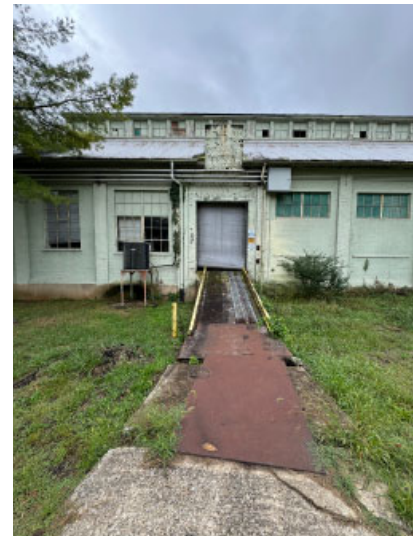
Typical mill brick pier wall construction. Section D has monitor at the roof ridge.
