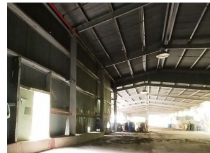
Section N: South side support beam, in bay to the right of doorway, is damaged.
