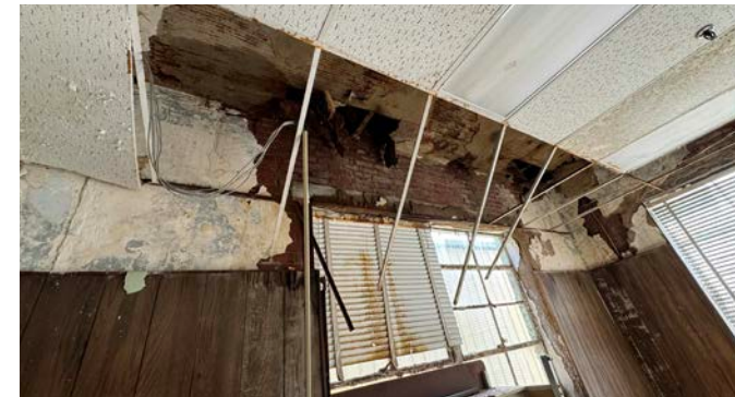
Water infiltration and damage in Section D.
