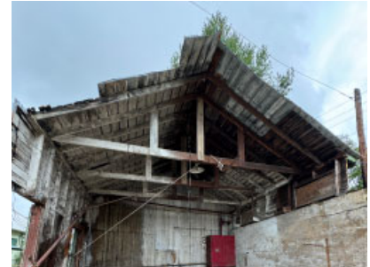
Building X: East end deterioration.
