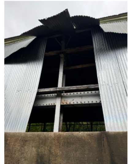
Section N: Metal wall panel condition.
