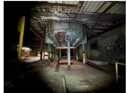
Section L: Existing tank on first floor, which extends into the second floor.
