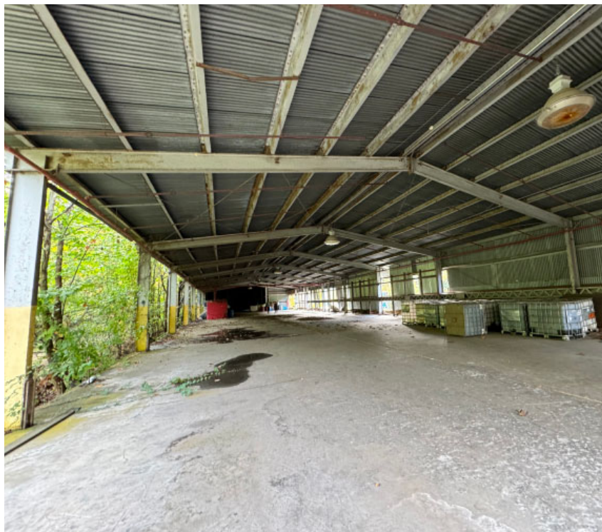
Section O: Looking east, with Section N at the far end of the structure.
