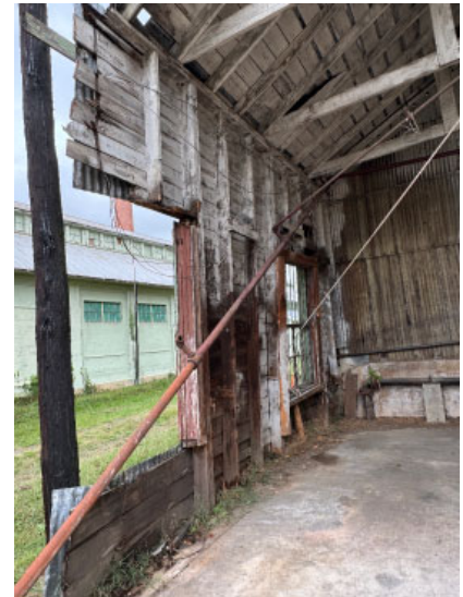
Building X: East end deterioration.
