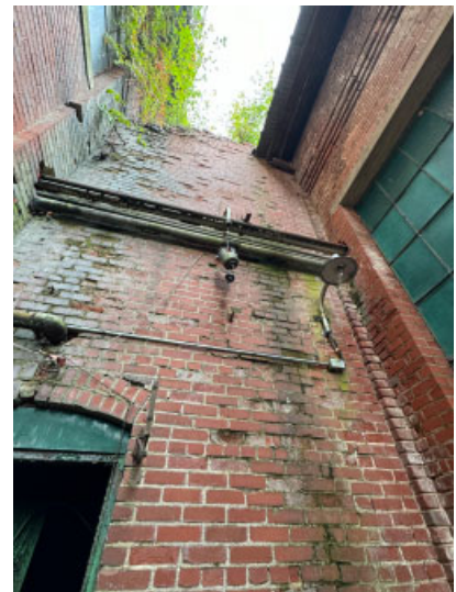
Section I, between Section G (left) and Section E/F (right): Masonry deterioration.
