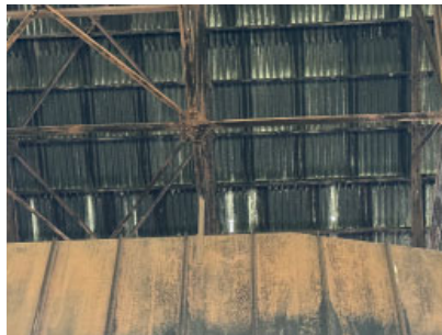
Section G: Typical roof condition, with exposed trusses and corrugated metal roof panels.
