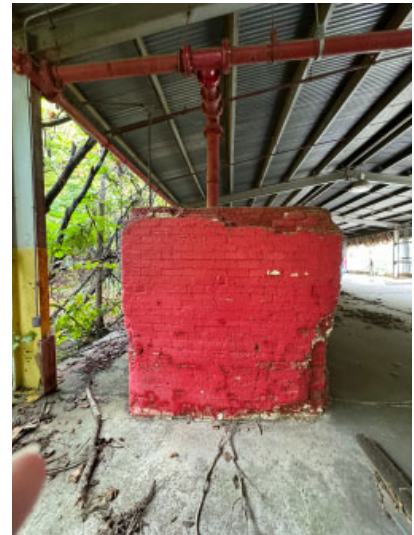
Section O: Sprinkler valve enclosure.
