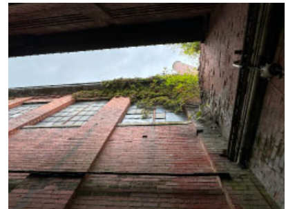
Vegetative growth and masonry deterioration at failed roof edge.
