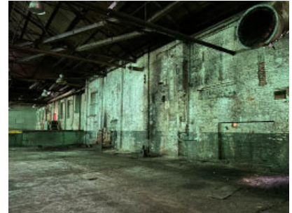
Section H: South wall. Elevated floor area of Section D visible in lower left corner.
