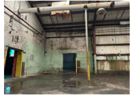
Section I: Southeast corner. The south wall is brick, then transitions to a concrete foundation wall with metal paneling above.
