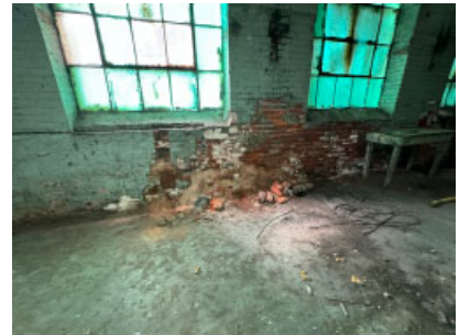
Section E/F: South wall masonry deterioration.
