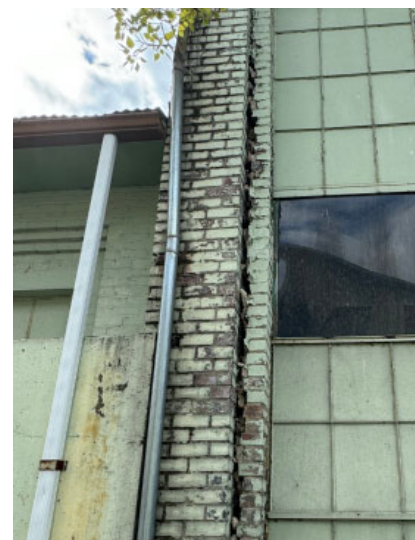
Section B: Pilaster failure on north wall.
