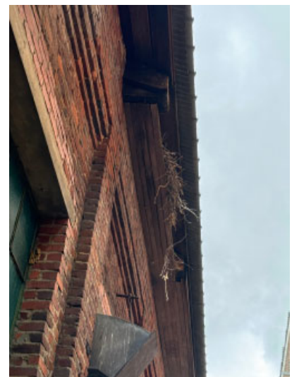
Wood soffit deterioration.
