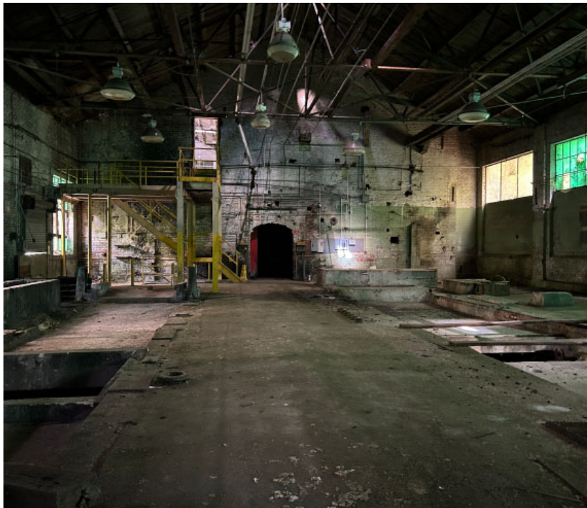
Section H: West wall, with concrete pits and curbs to the left and right.
