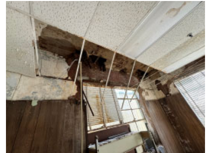
Interior deterioration of materials due to water infiltration at failed roof.
