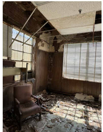
Section D: Southeast corner office condition.
