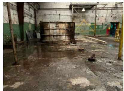
Water infiltration through roof openings.
